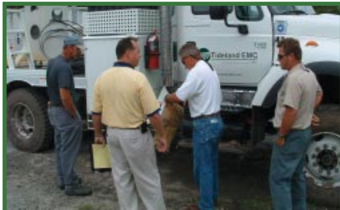
Tommy Greer inspects personal protective equipment on one of Tideland EMC's trucks, along with (from left) lineman Andy Midyette, safety director Wayne Brackin and Engelhard district superintendent Rodney Gibbs.
