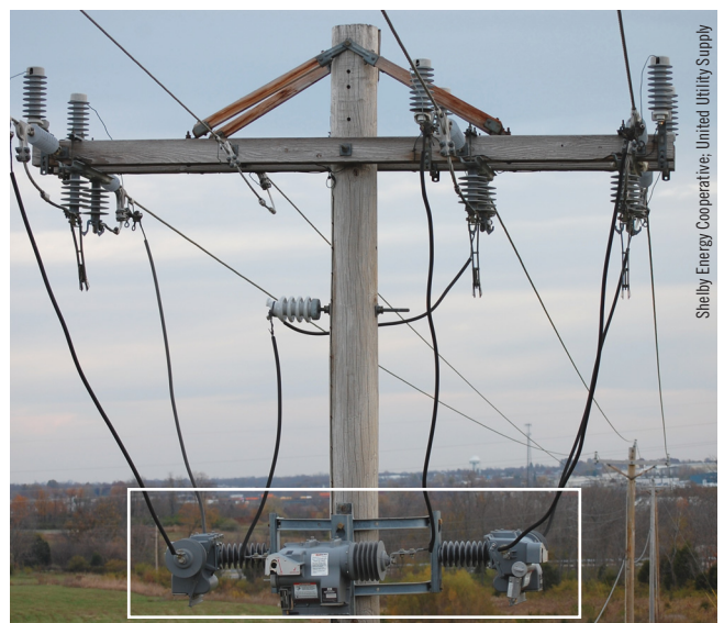
Reclosers protect lines and consumers from short circuits, and they allow temporary faults to clear, which helps keep service energized to the member without needless interruptions.
