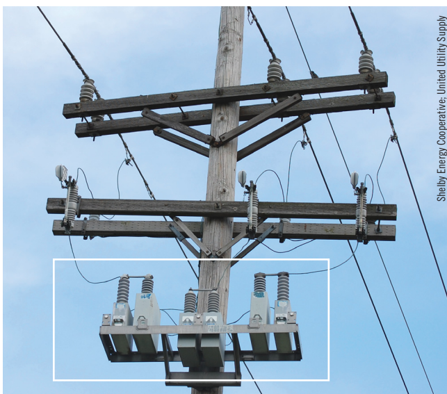
Capacitors improve the power factor on the utility lines—they prevent power from being wasted and help boost the voltage on long rural distribution lines.
