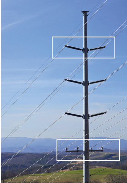
A Blue Ridge Electric pole carrying high-voltage transmission lines (upper) and lower voltage distribution lines (lower).
