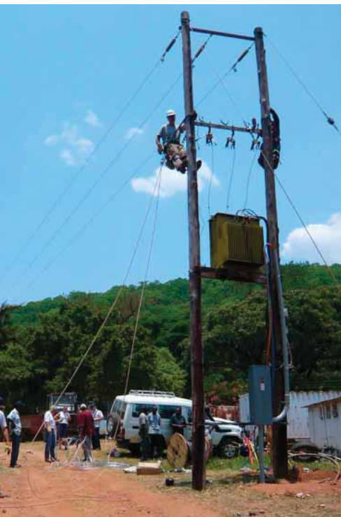
Ken Thomas worked with local lineworkers to rebuild distribution service to a hospital in Zambia.
