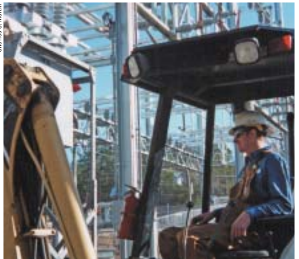
Photos this page: First-year lineman Clark Blackburn at work in a new Wake Electric substation.
