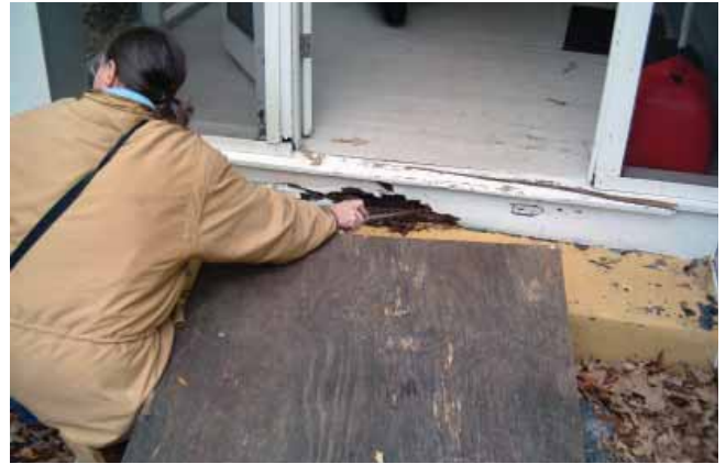
Evidence of rot at porch may point to more serious problems.
